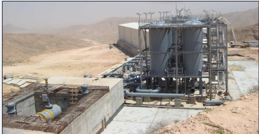
Valve Structure, Surge Vessels – Pump Station
