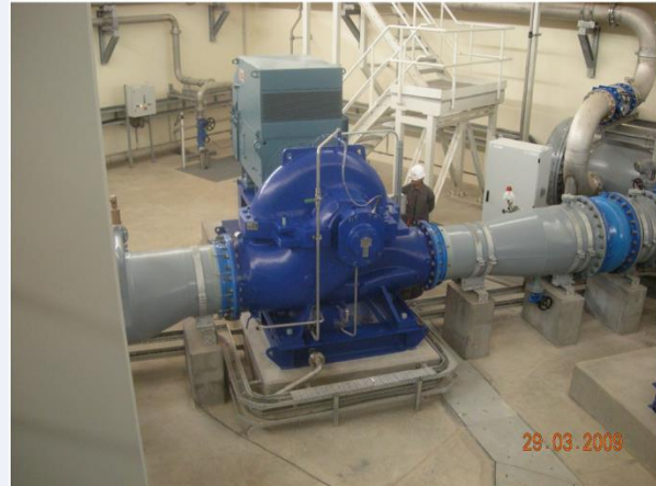
Pump and Motor Set
