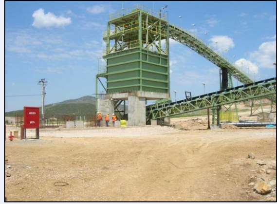
Secondary & Tertiary Crusher
