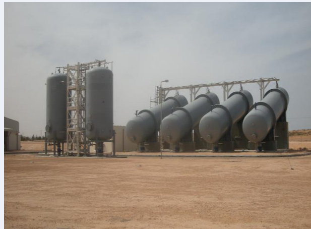
Outlet Surge Vessels
